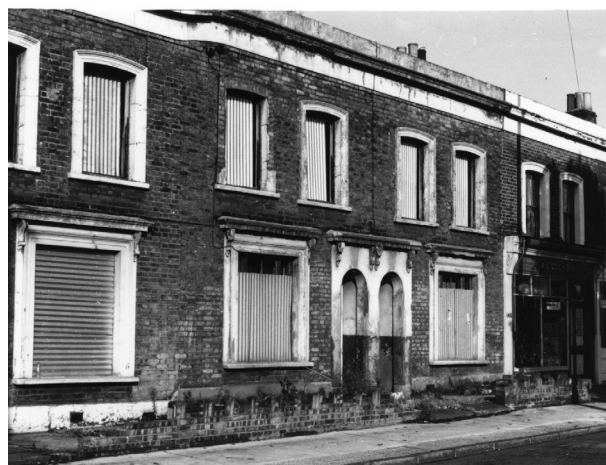
Boarded-up houses on Campbell Road, E3, awaiting repairs, Acme Studios (1974).
